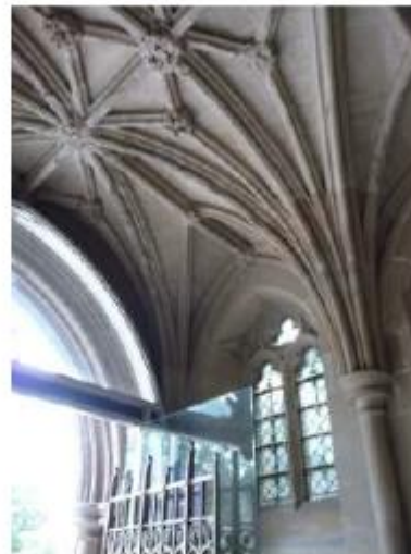
Vault within the Vaughan Porch and steel and glass frame for later doorway and screen.
